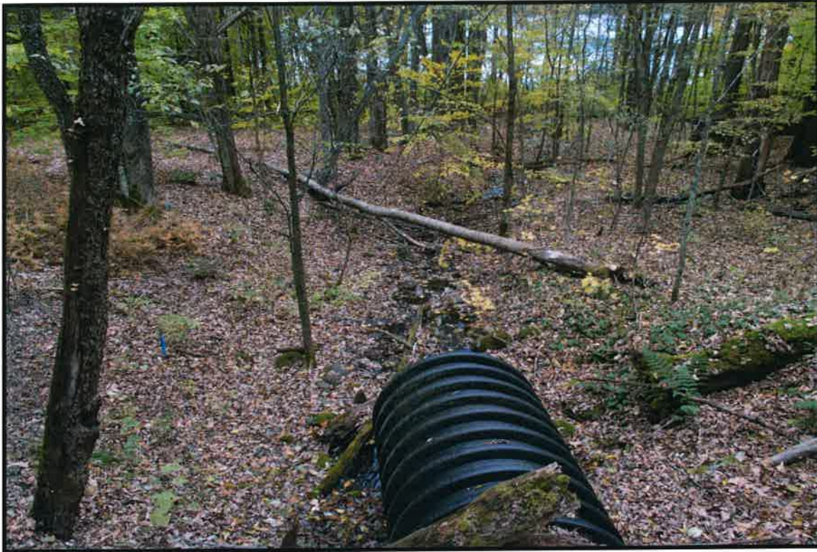
Photograph 11) View of the culvert and the intermittent stream that was identified as Area 18.
